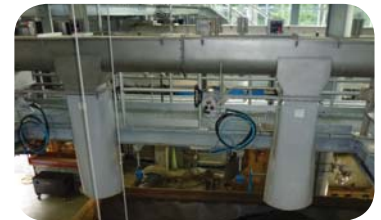
Truck outloading system
