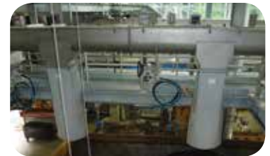
Truck outloading system
